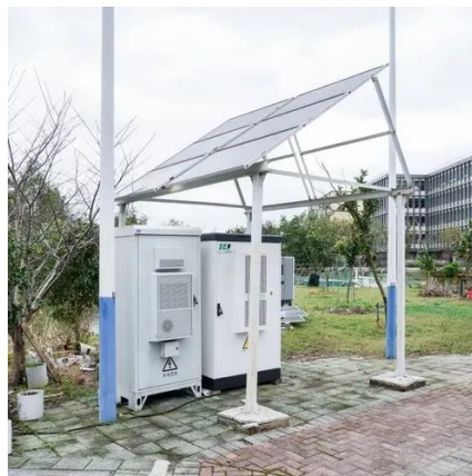
A solar park, solar farm, photovoltaic power station with trees and
