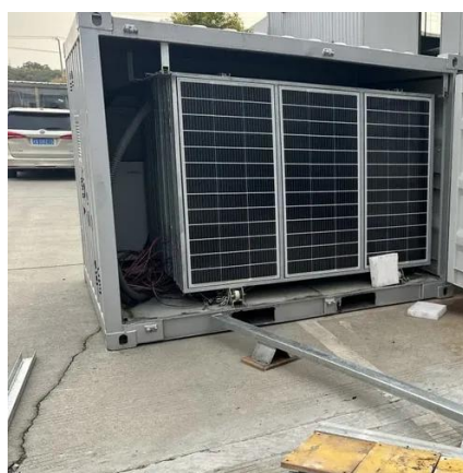
Photovoltaic power station
