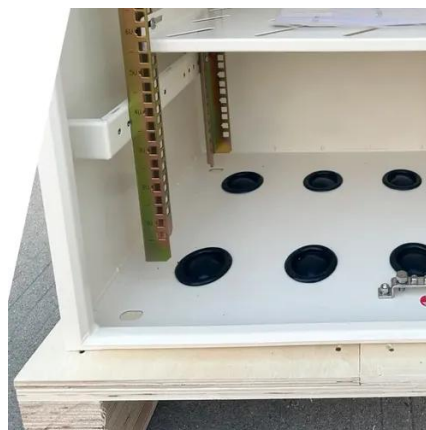
Inside Huawei's energy storage battery container
