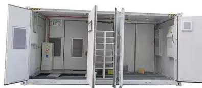
1075KW HH ESS
